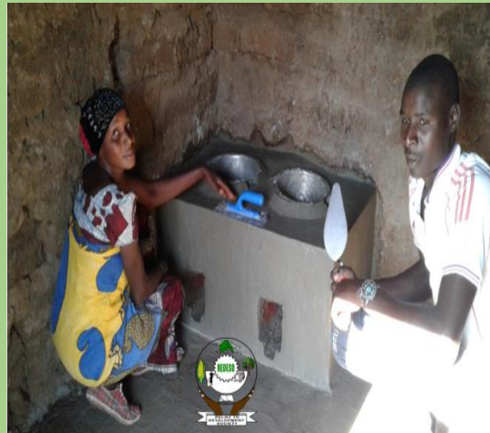
Photo 66 & 67: Youths trained and engaged in Construction of Cooking stoves as part of their day employment at Kiloleli village
