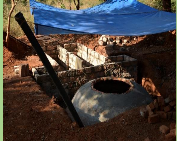
Photo 25: Fixed dome plastered inner and outer, fixed with high grade (Type "c") PVC for cow dung mixing chamber, outlet slurry chambers, to be connected to compost pit for horticulture gardening.
