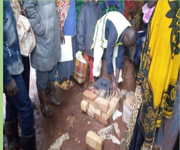
Photo 28: Repair of insert stove started with demonstrations of how to insert inside the burnt bricks binded with clay and lime mortar.
