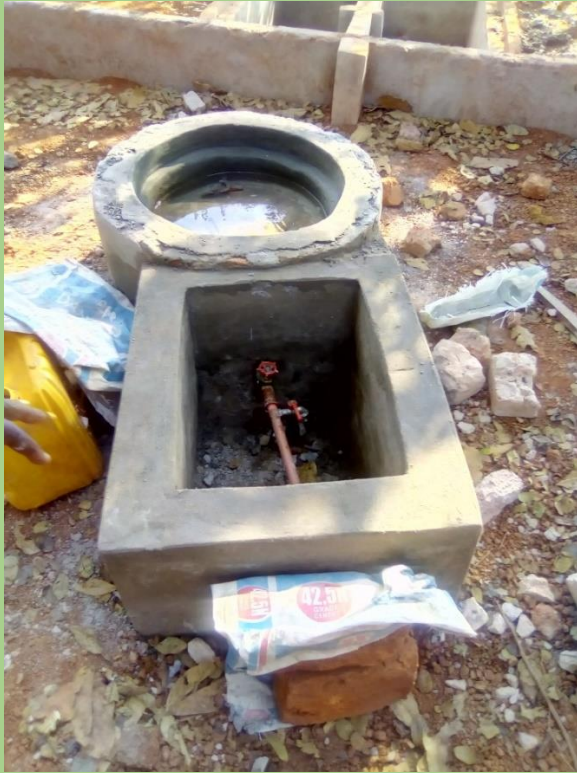
Photo 27: Water sealed chamber, with water for monitoring gas leaking, Gas outlet pipes fixed with gas control valves and system water trapped releasing tap.
