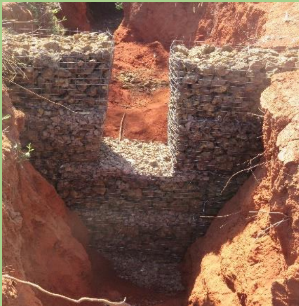
Photo 4&5: Conserved Water sources and soil erosion controls through the construction of gabion.
