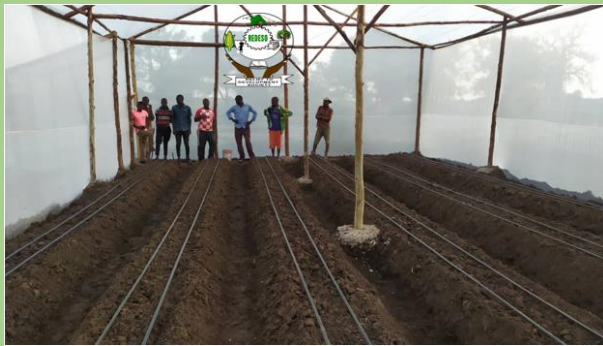
Photo 49: Group members observing the gardens ready for next step in one of the Constructed Greenhouses at Mihama and Ngundangali Villages
