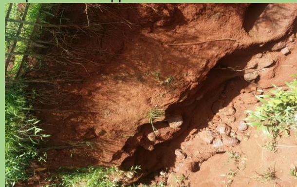
Photo 47: Gullies at zone 4 which needs rehabilitation, resulted in uncoordinated road construction.
