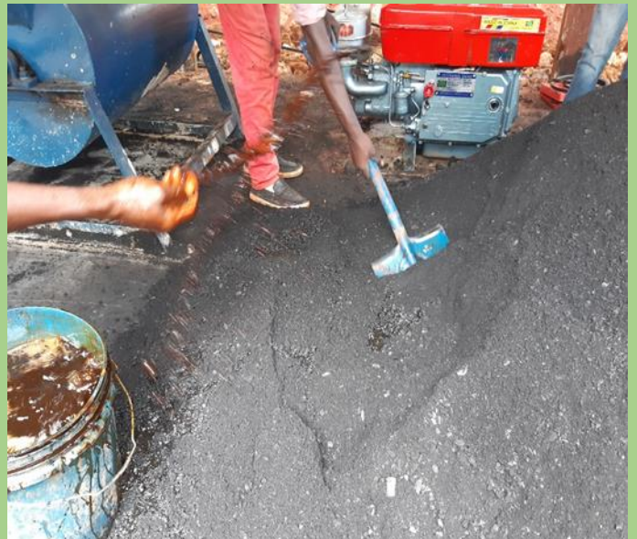
Photo 38: One of the Incentive workers mixing char powder and the binders in Nduta Camp.
