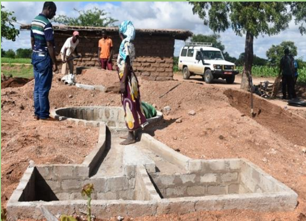
Photo 67: REDESO Project Coordinator (Charles Buregeya at left hand side) with Suzana Philipo and other working team having a progress checking up of the Biogas structure during final process of construction at Nhobola village.
