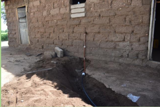
Photo 71: The connection of Biogas Pipes into Suzana's kitchen.
